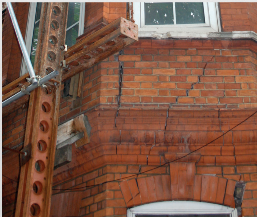
Severe structural damage caused by subsidence
