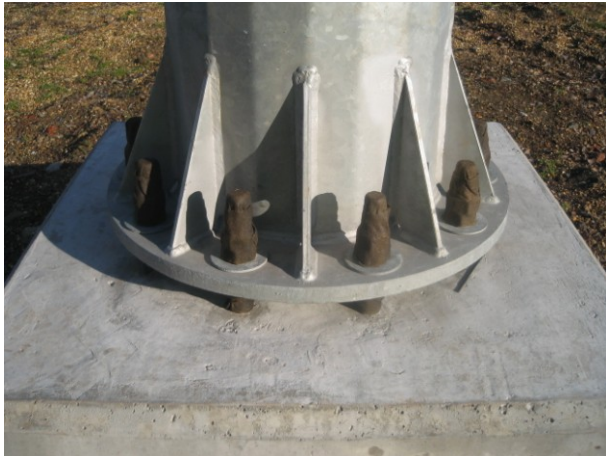
The plinth and anchor bolts for a high mast column.
