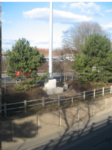
High mast installed between two carriageways on the A52.
